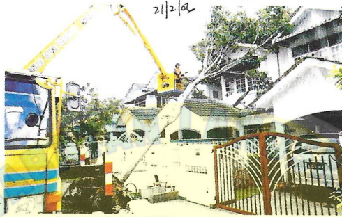
Contractors clearing the tree that fell onto a house in Bandar Kinrara, Puchong.
